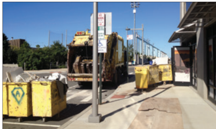
Demolition at The Stores at One Brooklyn Bridge Park. Photo by Lore Croghan
