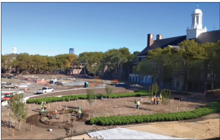
Visitors can visit the new $250 million park construction site at Governors Island this weekend only. Shown: Liggett Terrace. Photo by Trust for Governors Island
